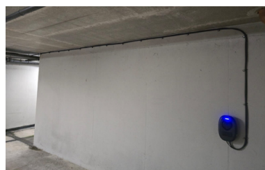
CHARGER CONNECTION POINT
