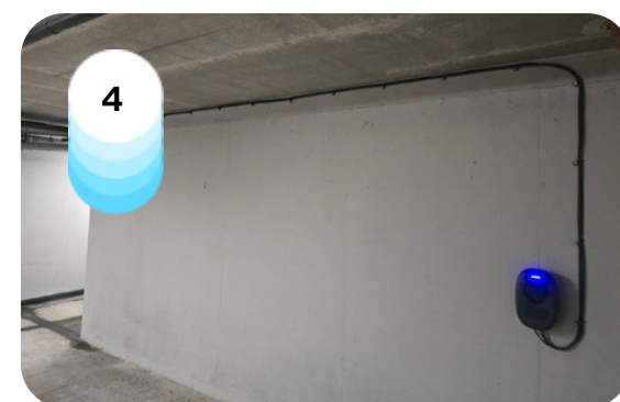
CHARGER CONNECTION POINT
