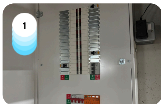
MAIN DISTRIBUTION BOARD
