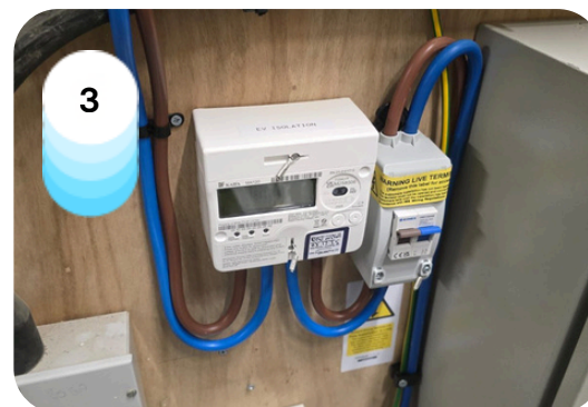
NEW DEDICATED EV SUPPLY
